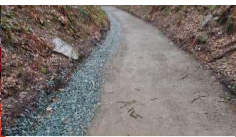
Completed the restoration of stretches of the Tamar Trails - after a kind donation of stone by Greystone Quarry
